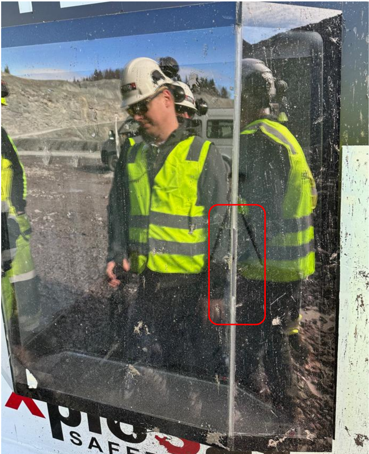
Image 6. The window without damage. The sealant holding 2 of the windows was slightly damaged. About 25cm of the sealant was blown away by the pressure.
